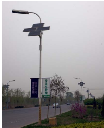
10 km of solar street lighting in Dezhou, China
